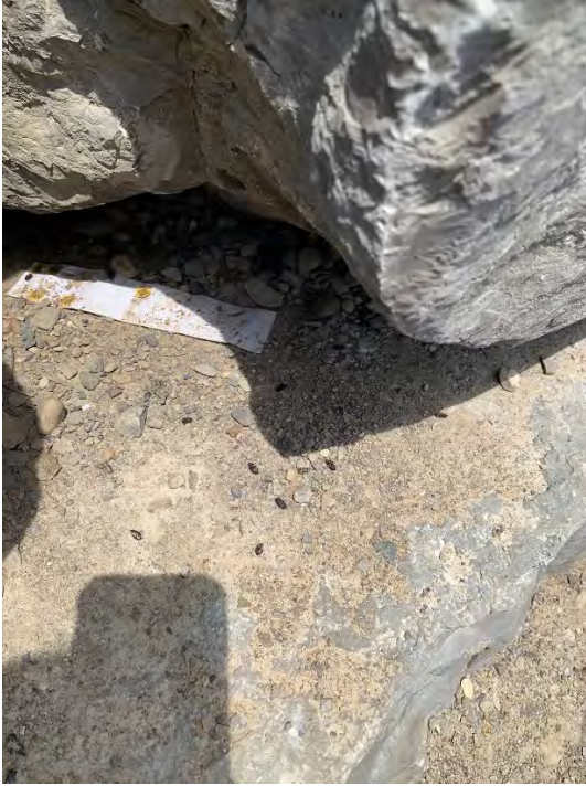
Photo of rodent feces observed along North wall – mid to west corner
