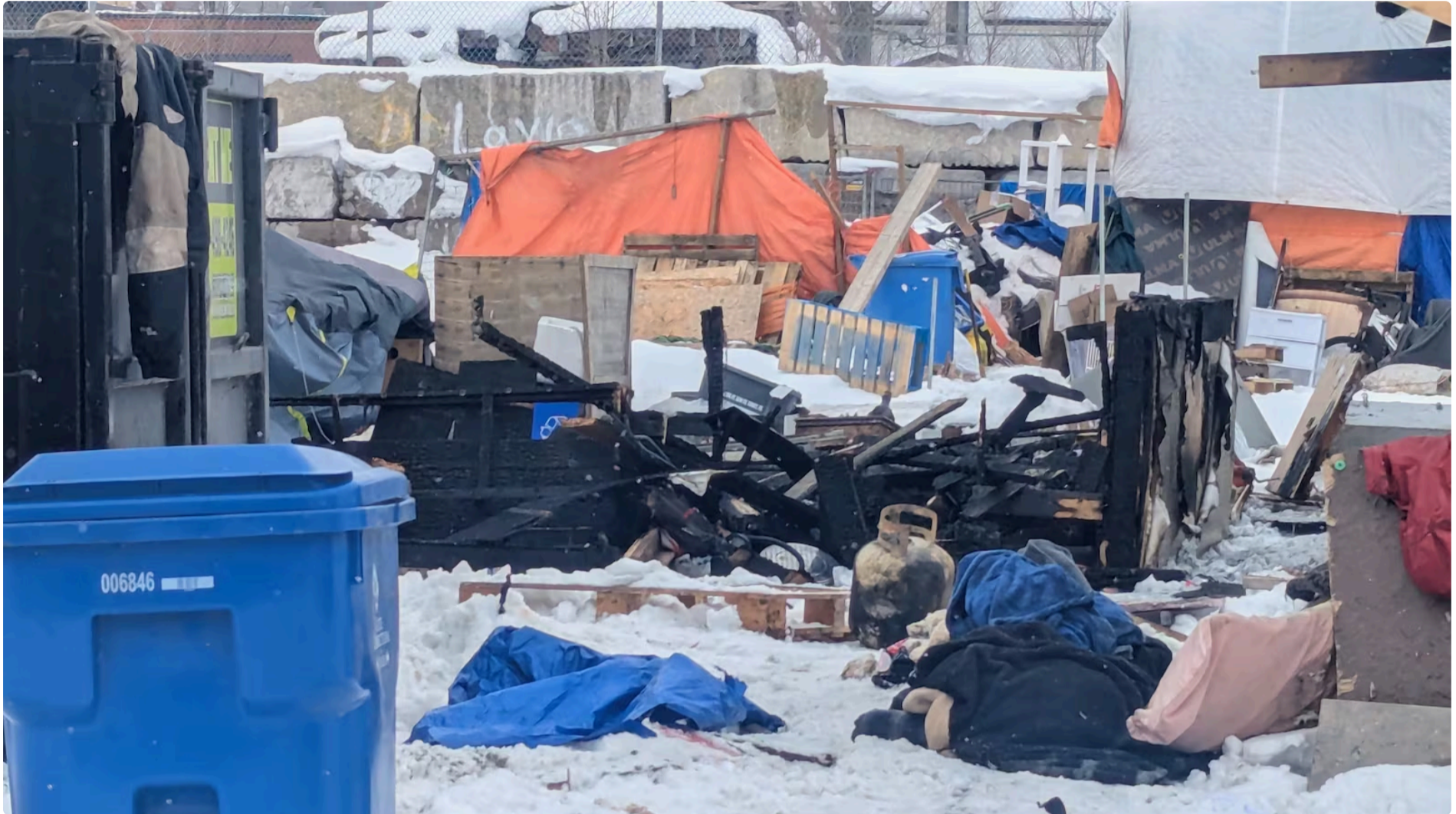
A damaged structure was photographed at 100 Victoria Street North in Kitchener, Ont. on Feb. 12, 2026. (Dan Lauckner/CTV News)
